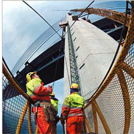
Engineers work on the Oresund Link Bridge. It was one of the most complicated structures ever designed using GT STRUDL. ( 300-dpi JPEG version - 856k )
